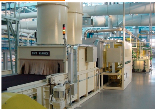
Continuous Operating CuproBraz® Furnace.
